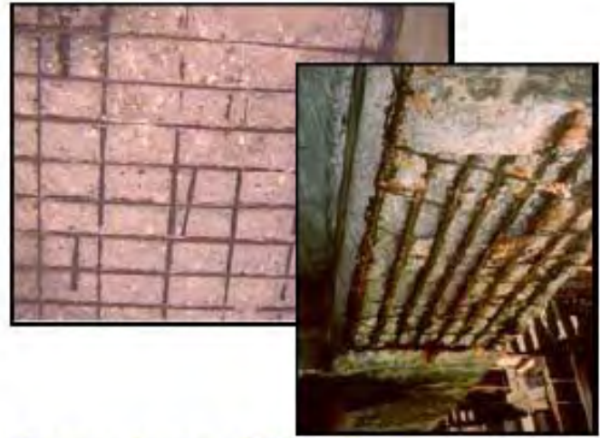
Corrosions of Steel reinforcements
